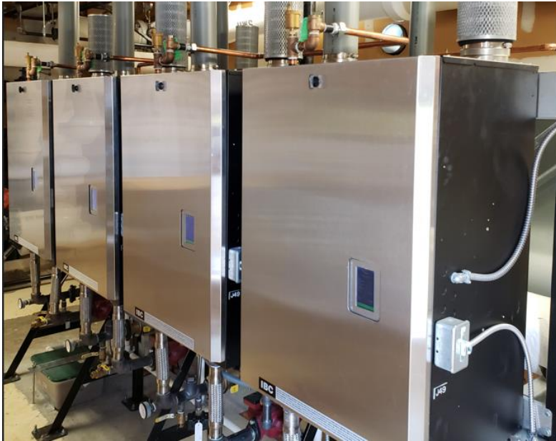
Figure 1: Four of the IBC boilers
