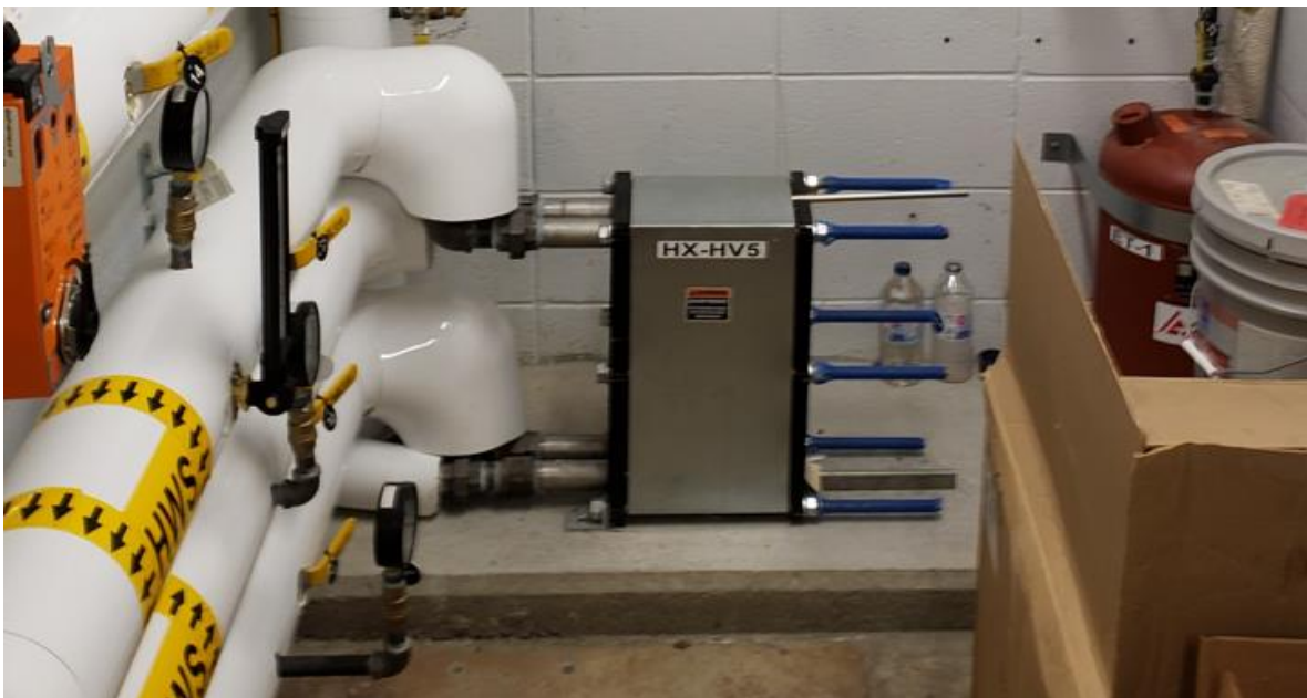
Figure 4: HX-HV5 heat exchanger
