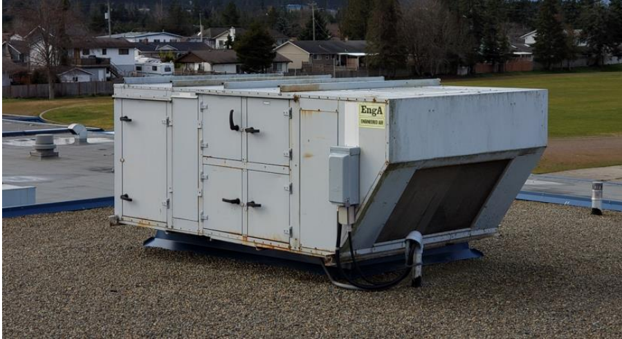
Figure 28: HV11A rooftop unit with DX cooling
