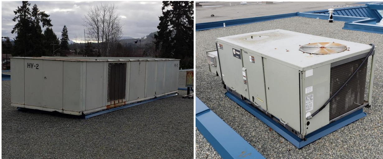
Figure 27: HV2 and HV4 rooftop units with DX cooling
