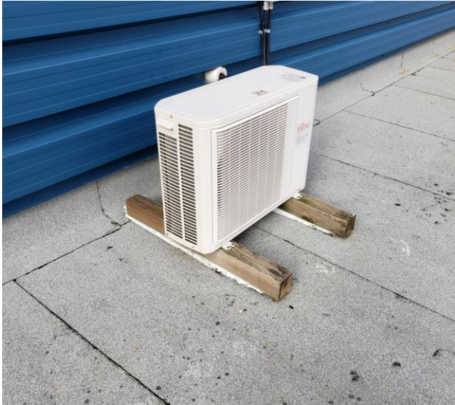
Figure 5: Additional Fujitsu split unit above multi-use area.
