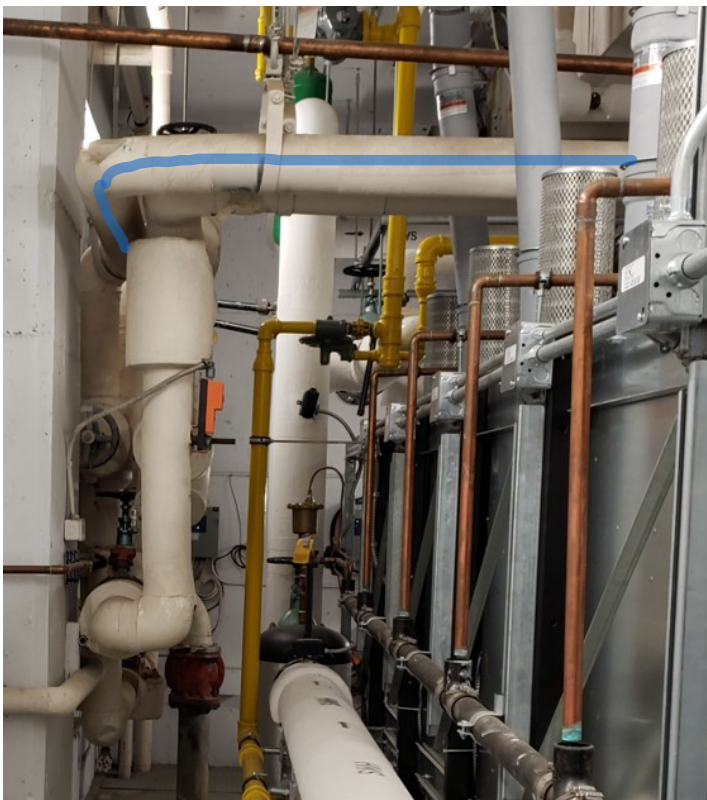
Figure 28: Basement mechanical room. Chiller water pipe marked in blue. The boilers are on the right.
